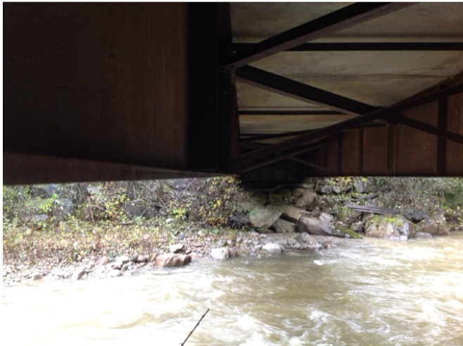
both girders have slight undulations in the bottom flange where the girders were welded
